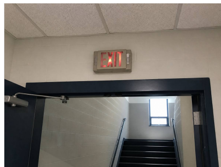
Photo 2 — Main Academic Building – East Stairwell — Emergency + Exit — 2026-07
