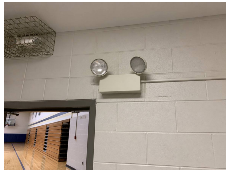
Photo 1 — Gymnasium – West Exit — Emergency Light — 2026-07
